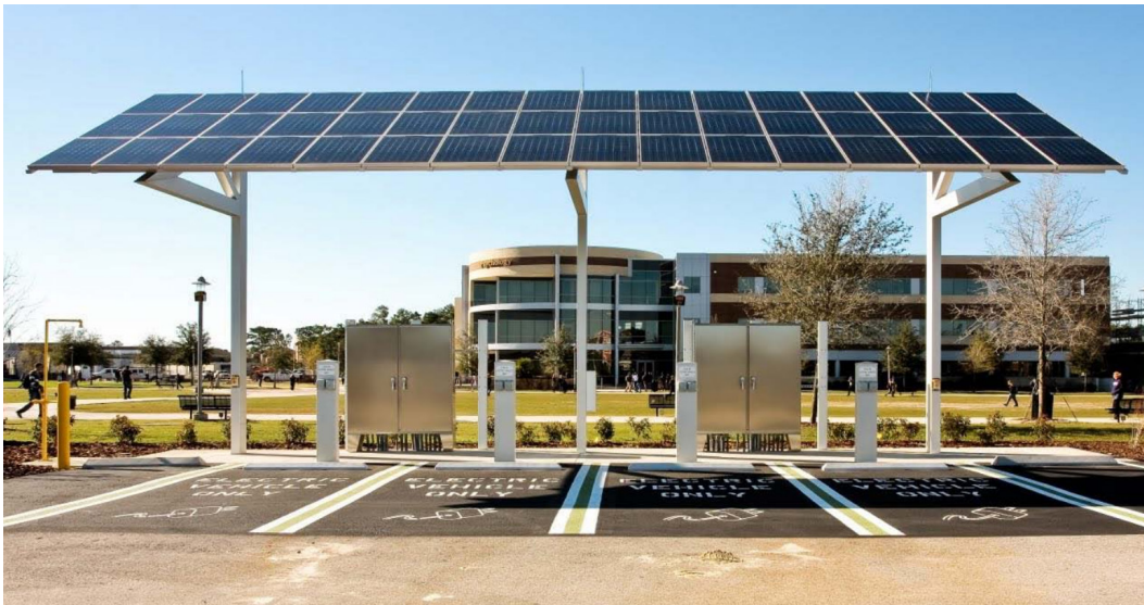
Figure 3-6. Electric Vehicle Charging Station with Solar Generation [52]
