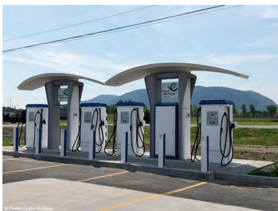
Figure 2: Super-station charging station (Source: Government of Québec)
