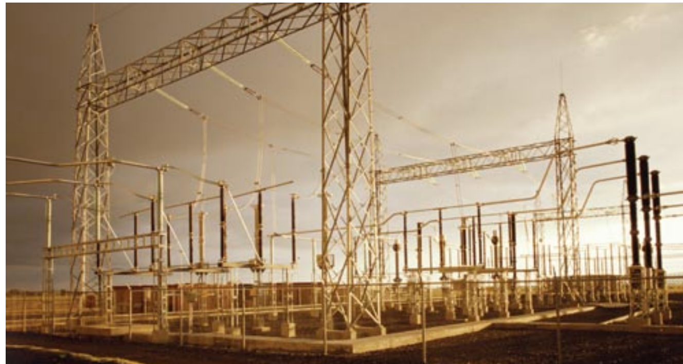
Pylons at a power generation plant.
